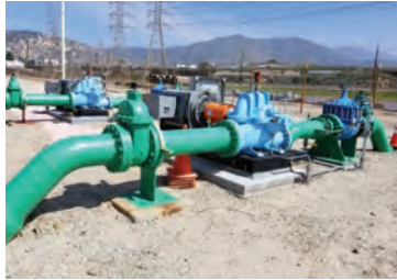
The new pumping units 1 and 6 at the Penstock Pump Station in Granada Hills help increase reliability, redundancy and capacity of water supply.
