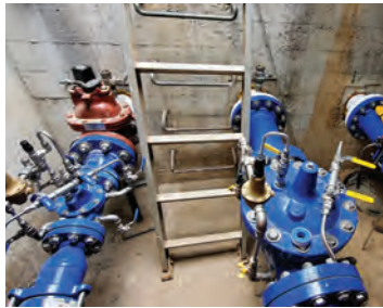
The Villa Woods Regulator Station in the Pacific Palisades area serves as a supply and pressure regulating station.
